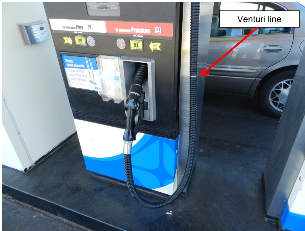
Photograph # 2: Nozzle # 20 hose showing venturi line as installed during inspection.
