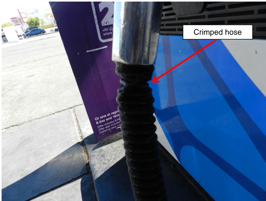
Photograph # 4: Nozzle # 8 hose crimped.
